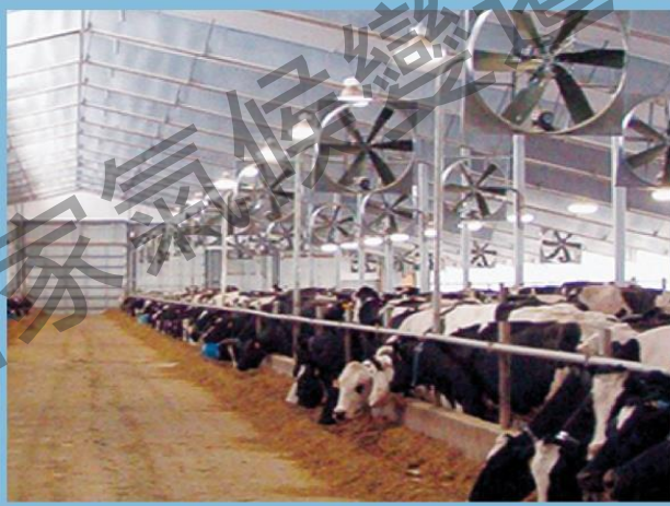
Moderate cooling Open Barn with Fans
