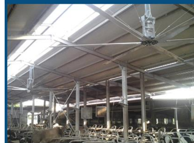
Intense cooling Barn with Air Conditioning
